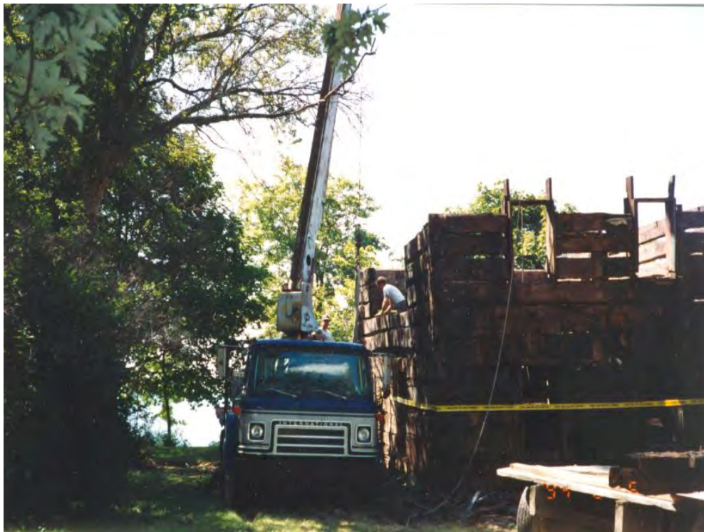
Plate 13: Portion of the Hoover Log Cabin that remained following the fire in 1994
