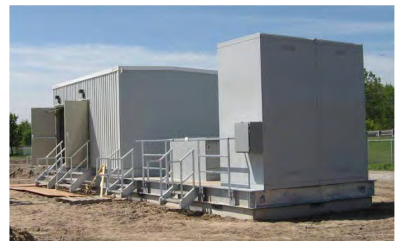
PV Interconnection Switchgear
