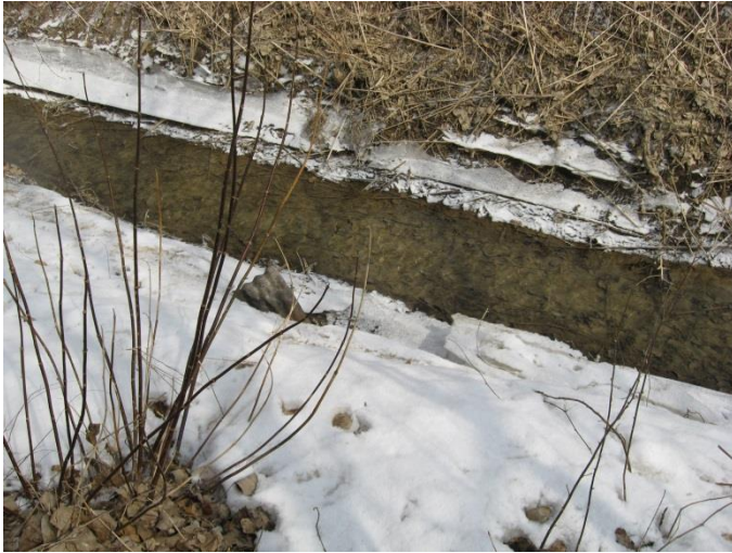
Photograph 5. ↑ Location of culvert draining out into watercourse east of and behind pond.
