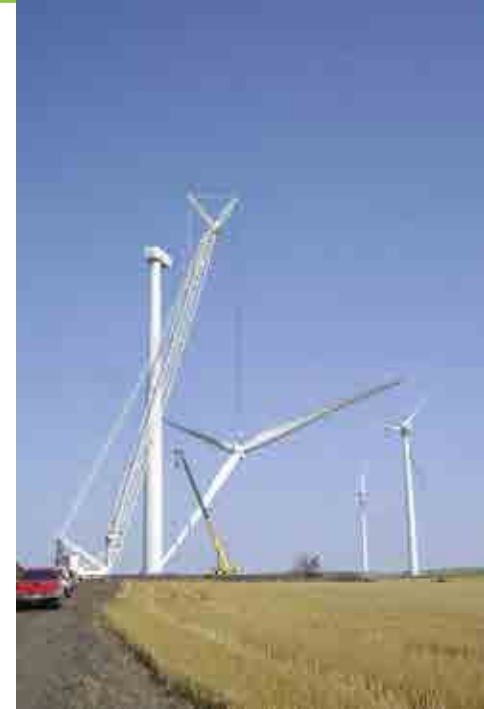
Cranes lift a rotor to be installed on the nacelle at the top of the tower.
