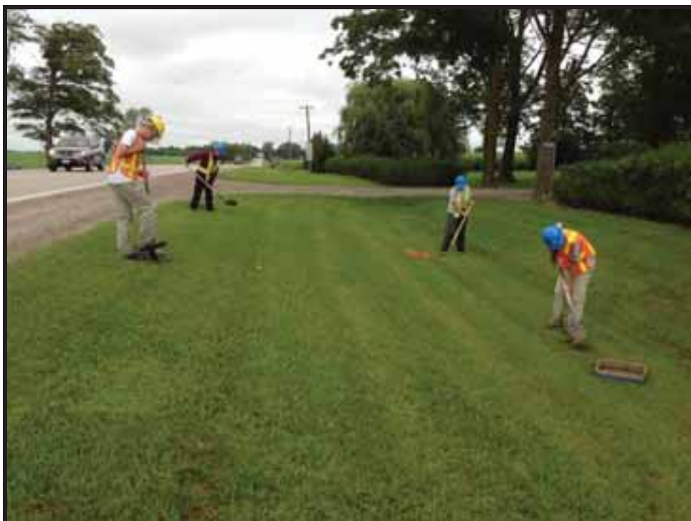
Image 34: View of Crewmembers Test Pitting to Confirm Disturbance at BLW1069 (Photo Taken August 8, 2013; Facing North)
