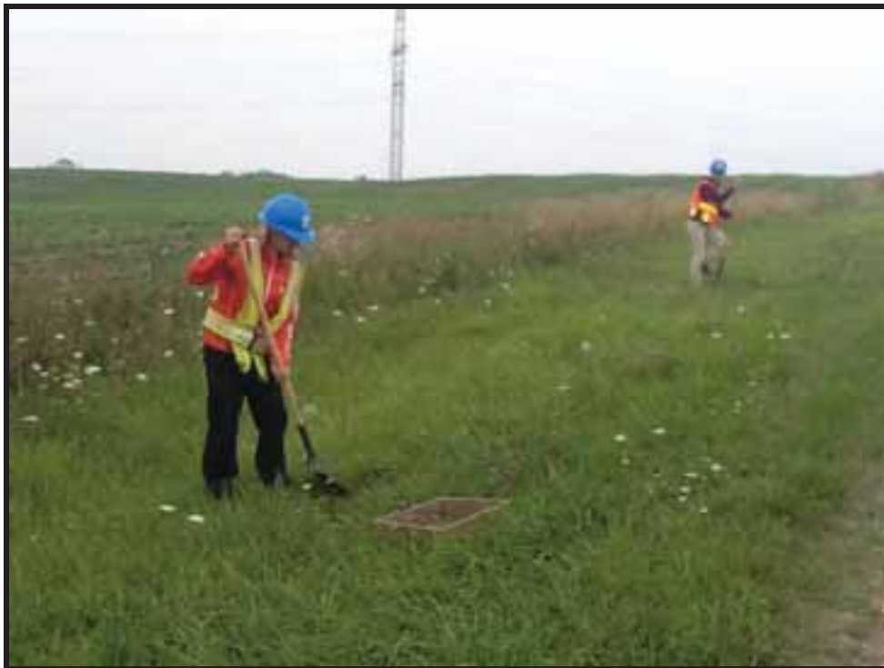
Image 86: View of Crewmembers Test Pitting to Confirm Disturbance at BLW1671 (Photo Taken August 6, 2013; Facing East)
