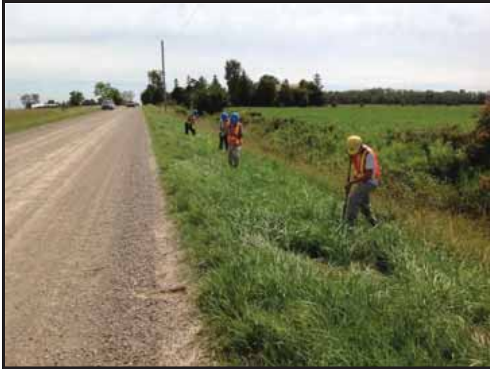
Image 97: View of Crewmembers Test Pitting to Confirm Disturbance at BLW1845 (Photo Taken August 8, 2013; Facing South)
