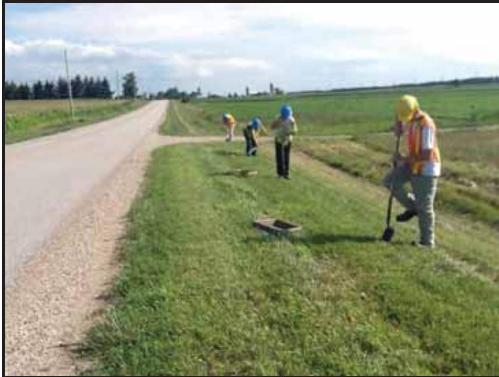
Image 25: View of Crewmembers Test Pitting to Confirm Disturbance at BLW1058 (Photo Taken August 7, 2013; Facing South)
