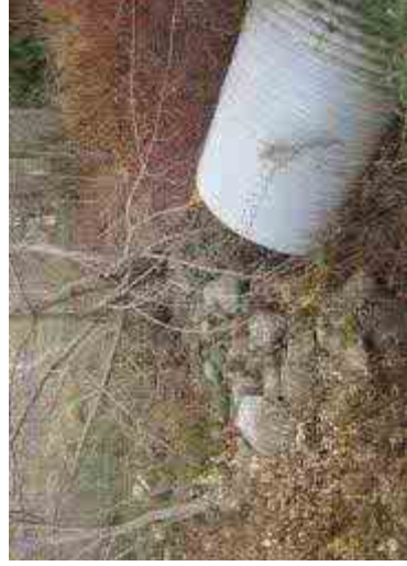
Photograph 2. Buried channel on east side ↑
