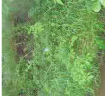
Photograph 3. Bank slumping on North side ↑
